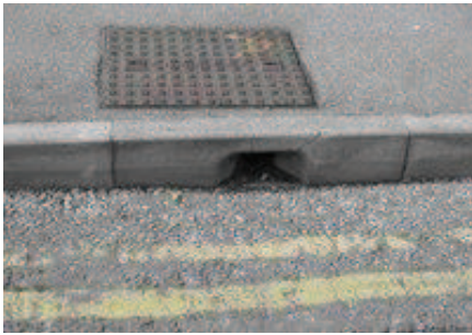
Typical Side Entry Gullies
